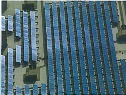
Solar Panel Array on Warehouse Roof
